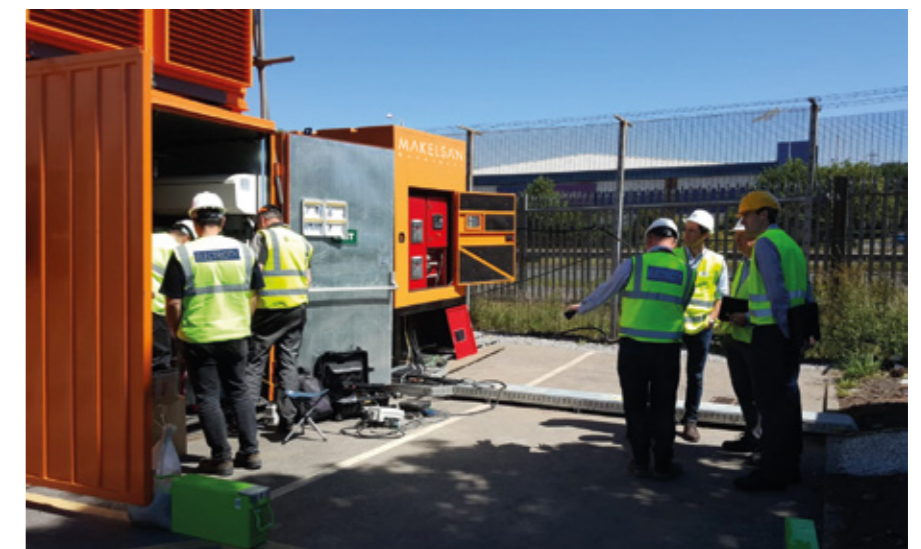
Electricity Northwest Whitbirk Plant, where DRM is installed - National Grid Tests
